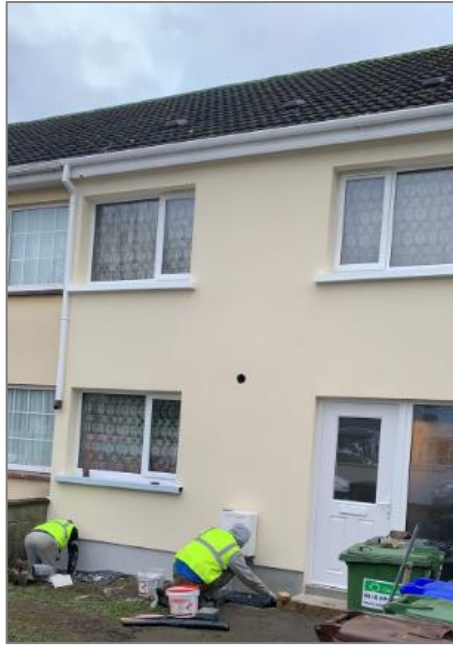
Figure 3.11: Retrofitting of housing with improved insulation, doors, windows, and heat pumps to improve energy efficiency in Carrig Glen, Blessington.
